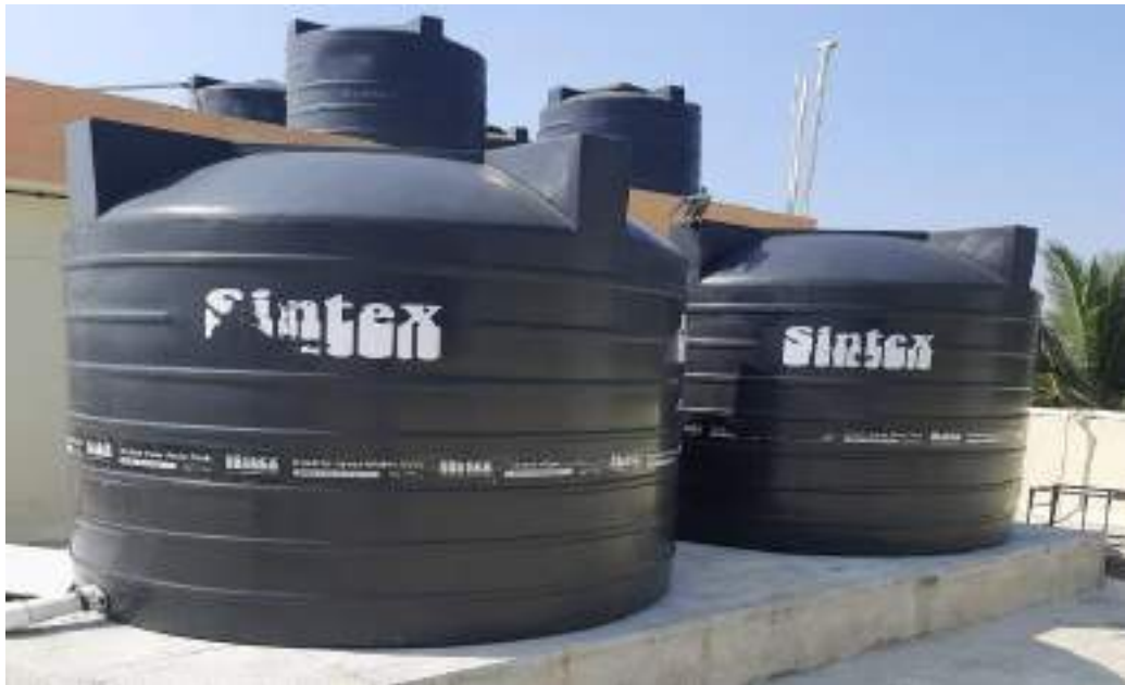
Figure 11: Syntax tanks for Fire Safety Systems
