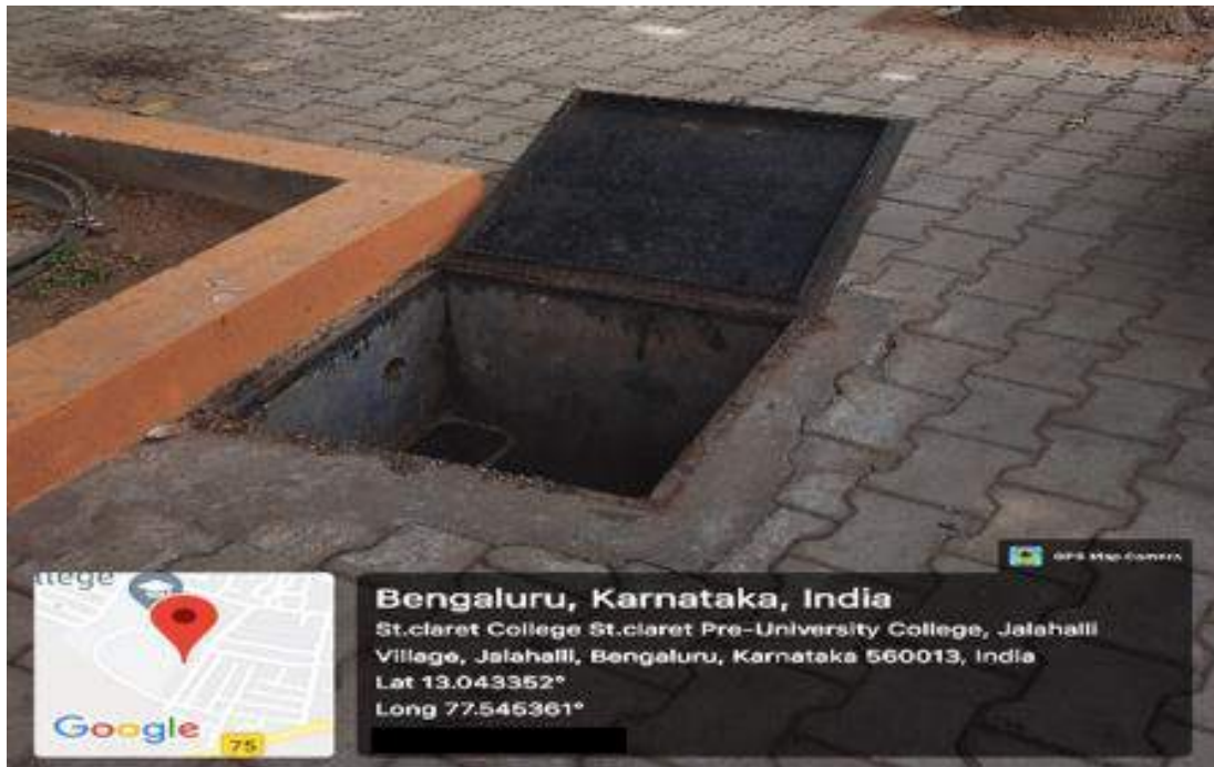
Figure 13: Underground Storage Tank for Rainwater
